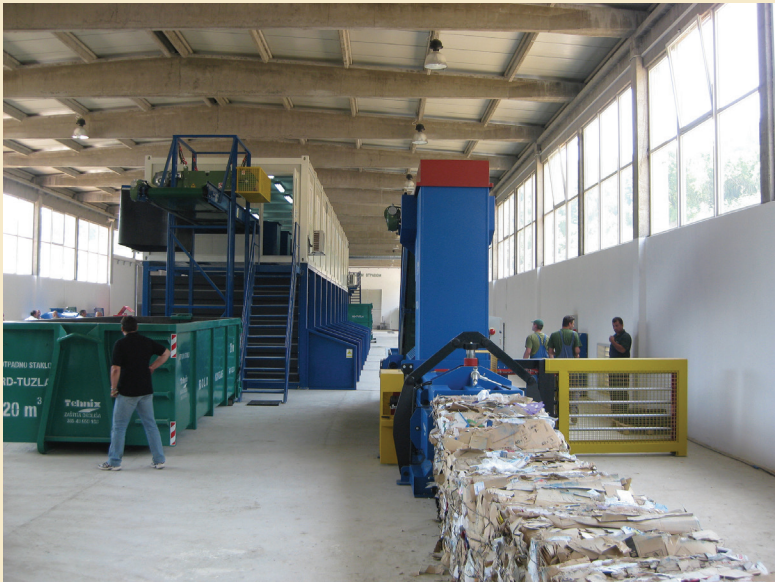
Photo 3.3 Recycling Plant in Bosnia and Herzegovina
