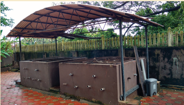
Photo 7.7c Decentralized Composting Units in Panaji, India
